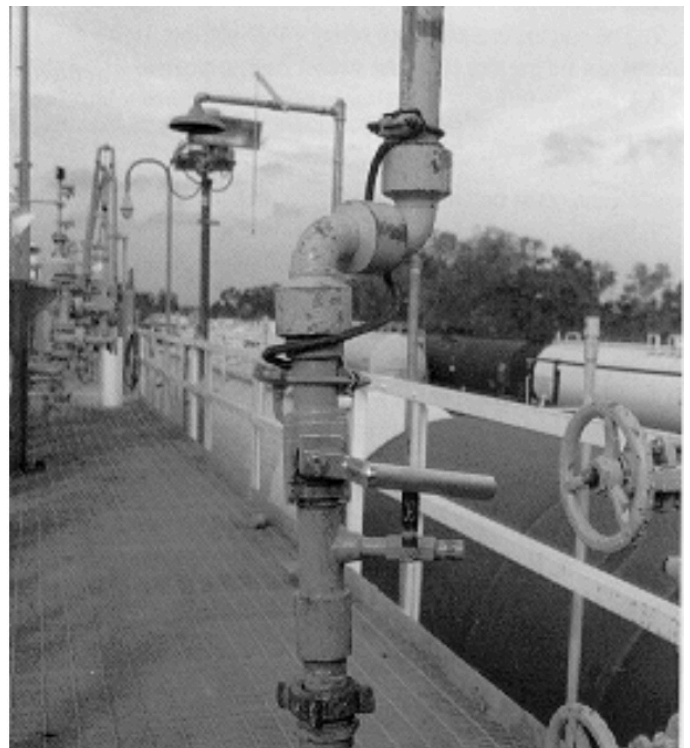
Close-up of end of loading arm fittings, showing valving that allows purging prior to disconnecting, threaded fitting for connection to tank car valve and bonding wire around loading arm swivel joints.
