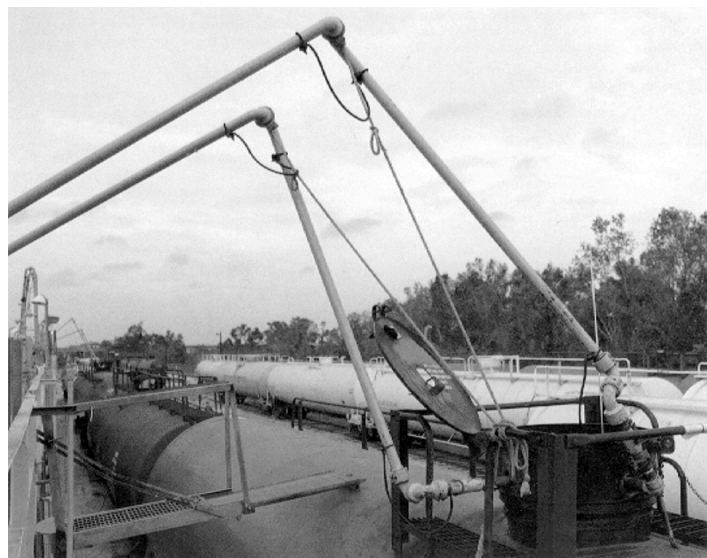
Typical butadiene rail tank car loading, showing liquid vapor connections. Magnetic gauge stick is visible.
